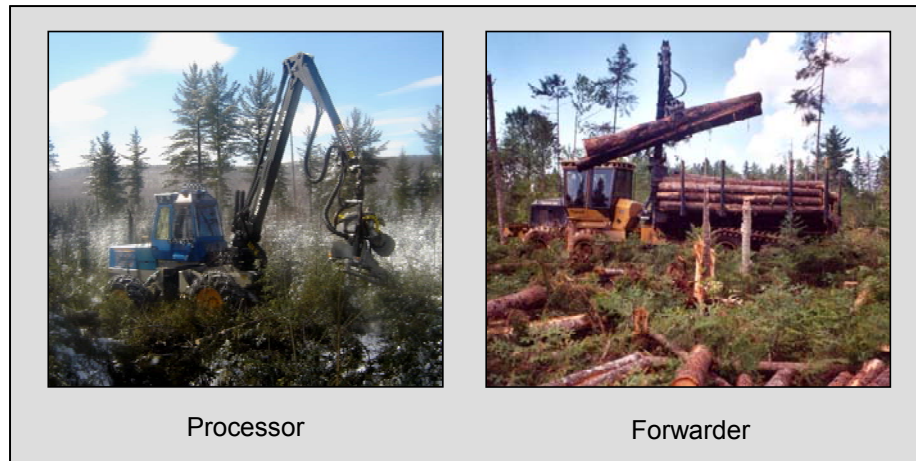
Figure 15: Cut-to-Length System Equipment 12
